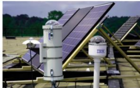
Solar panel power converter
